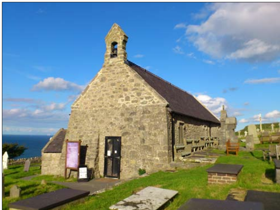
St. Tudno's Church after refurbishment. Note the new pointing on the upper gable.
