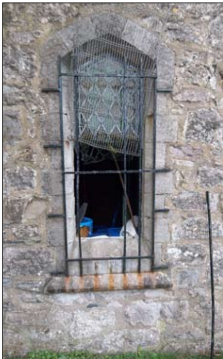
The broken vestry window.
