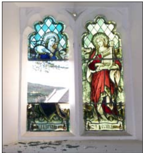
The damaged window to St. Miriam.
